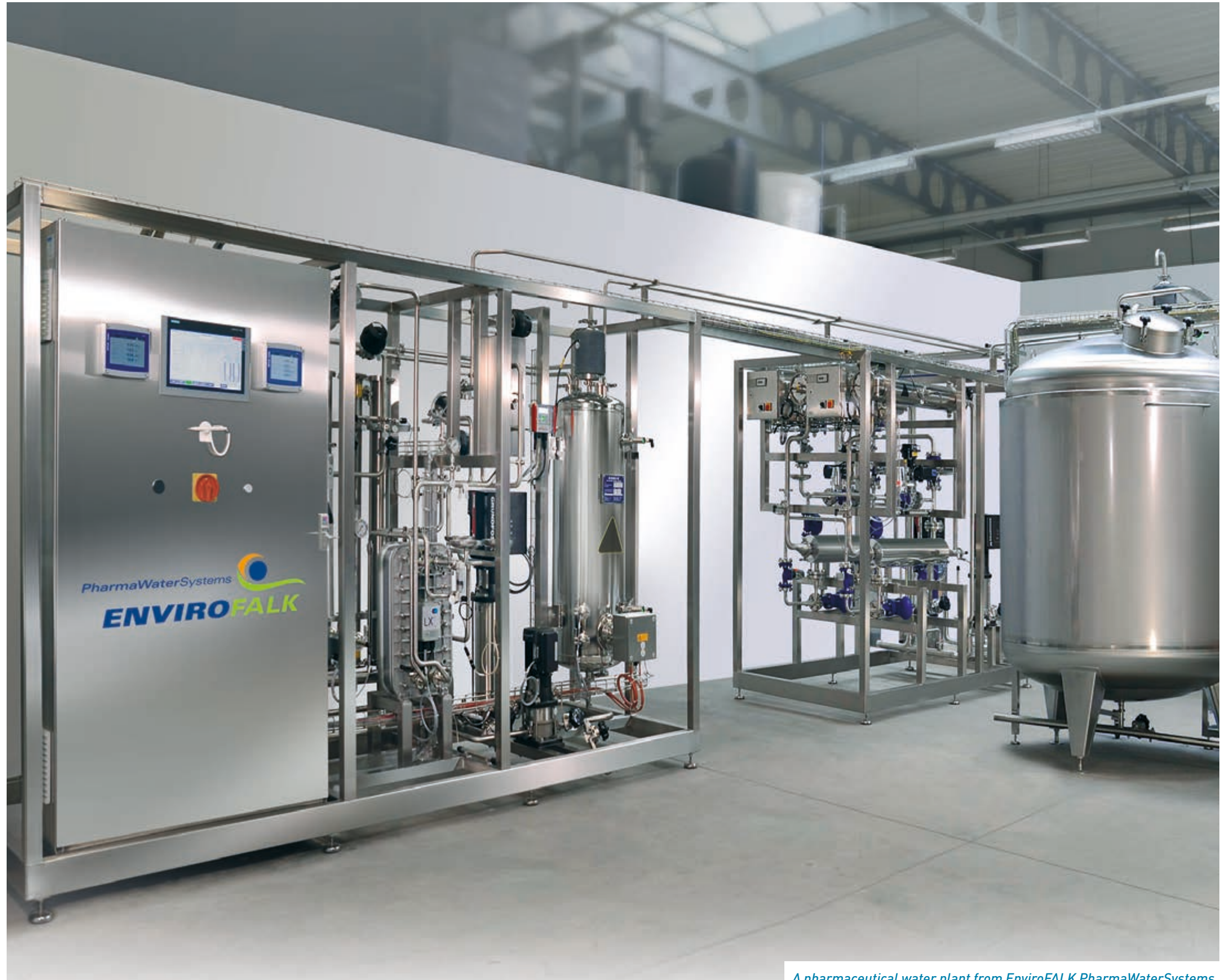
A pharmaceutical water plant from EnviroFALK PharmaWaterSystems
